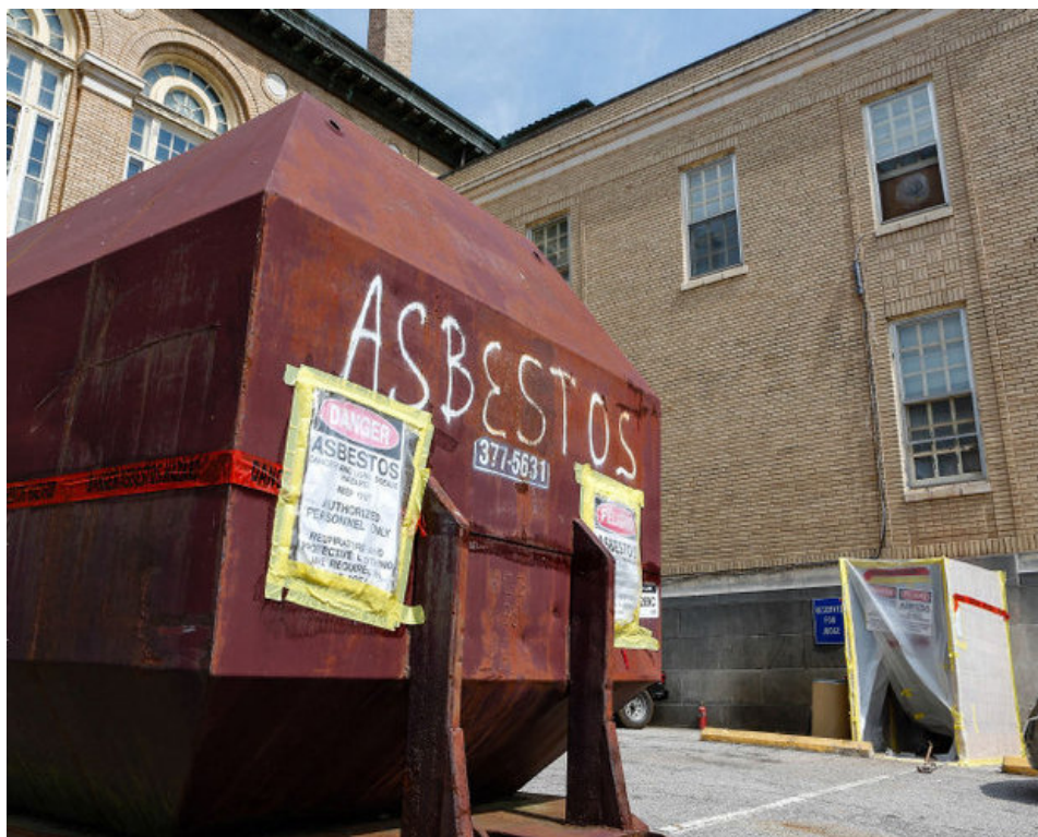
Large containment unit stands next to the Courthouse as asbestos abatement is underway at the York County Courthouse in York.
